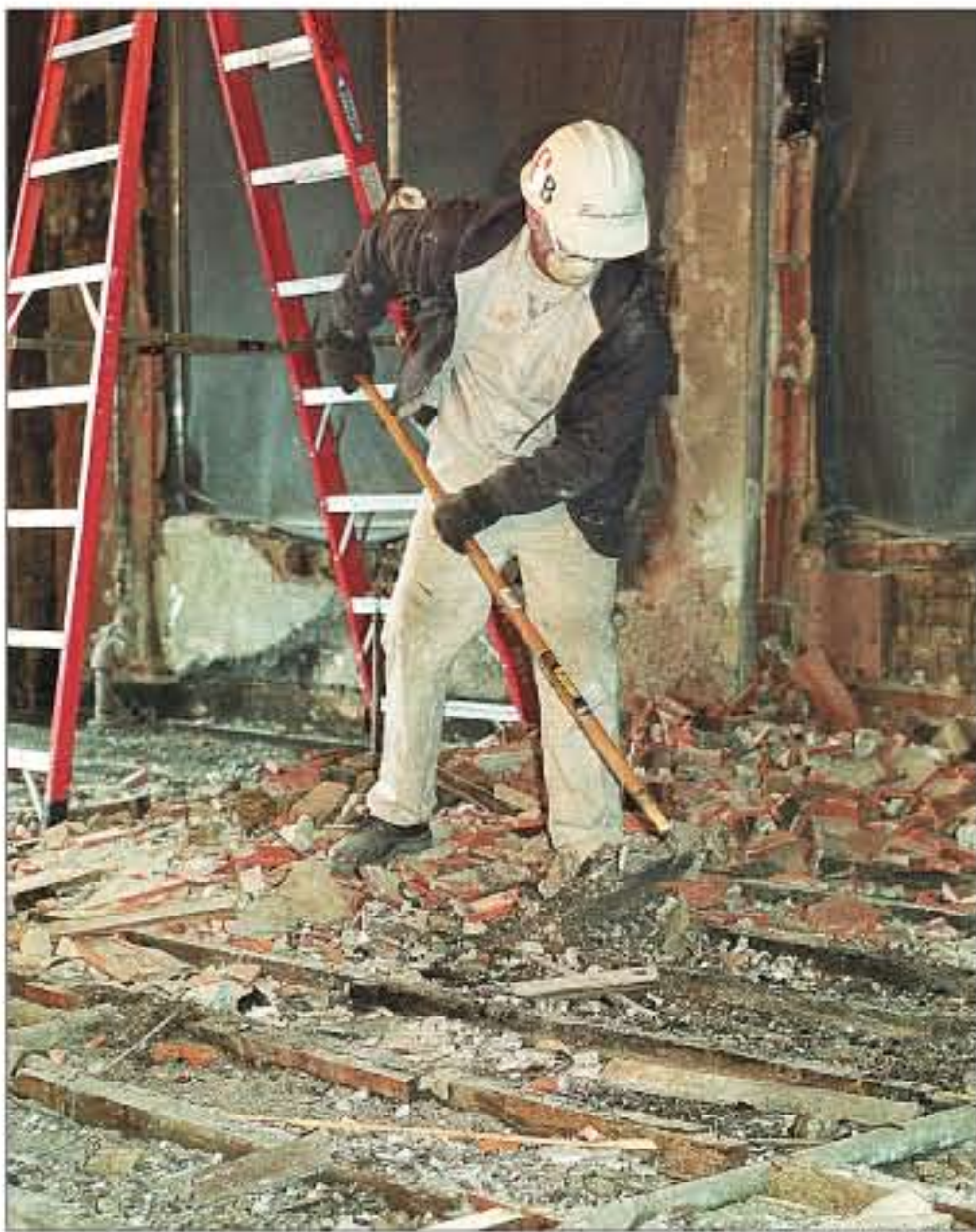
Stan Clayton of Burton Brothers cleans the rubble of the Institute of International Agriculture's offices in Agriculture Hall on Jan. 13, 2000, after a suspected arson damaged the rooms.
